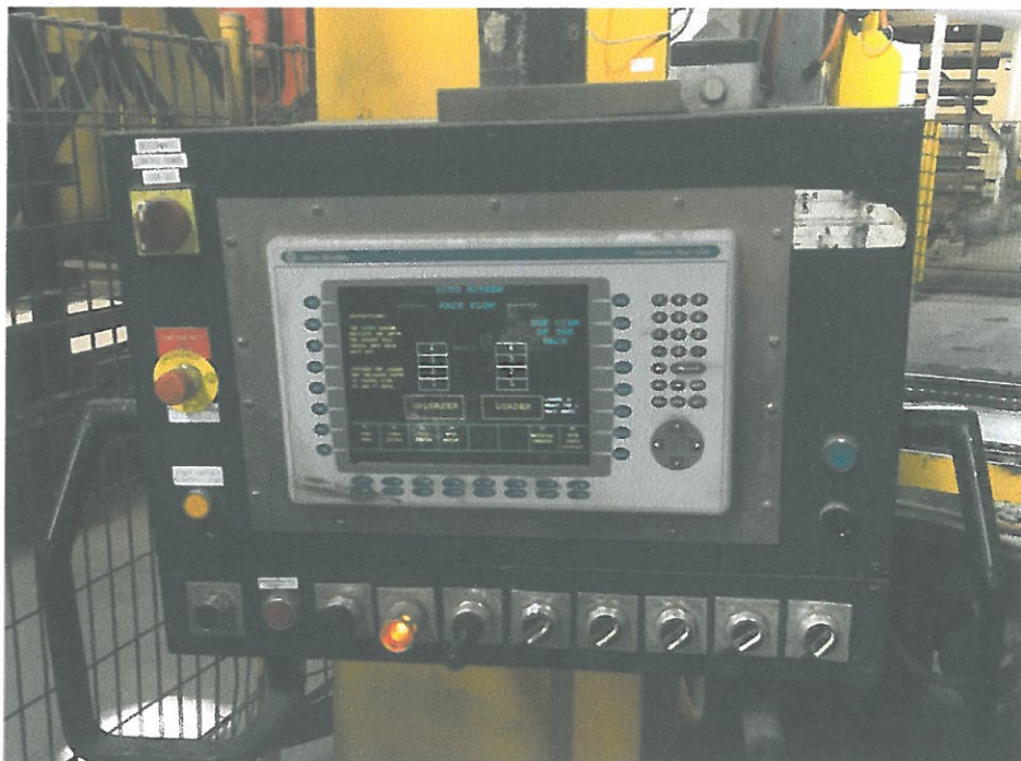
Bessermatic control panel
