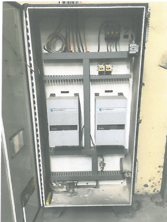
Smartpac electrical panel
